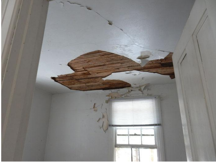
Figure30: 200 John Street, Garage, Ceiling Damage
