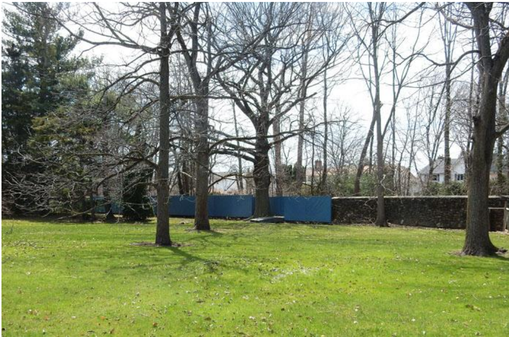
Figure92: 588 Charlotte Street, Cobblestone Wall on Railway Trail, Wooden Replacement Where Wall has Collapsed
