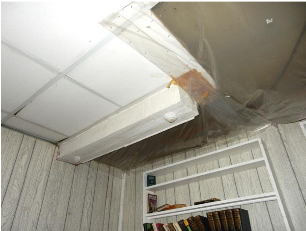
Figure 35: 200 John Street, Garage Apartment, Beaver Board Walls, False Ceiling and Ceiling Damage
