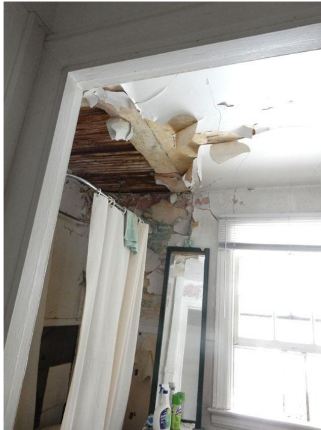
Figure 31: 200 John Street, Garage Apartment, Bathroom Ceiling Damage
