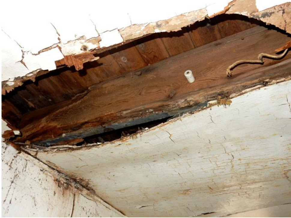
Figure58: 200 John Street, Pool House, Ceiling Damage
