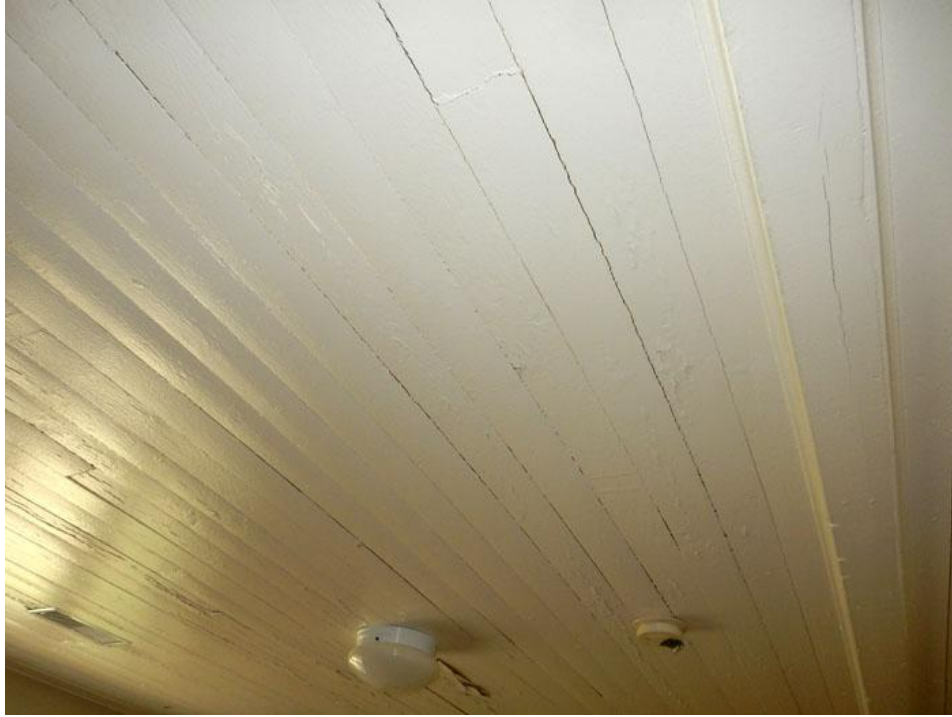
Figure80: 588 Charlotte Street, Stables/House, Apartment Bedroom Ceiling
