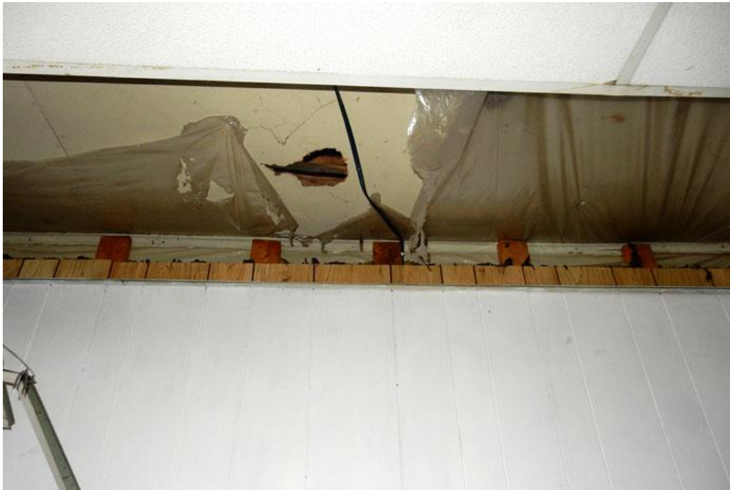
Figure 33: 200 John Street, Garage Apartment, Bedroom Ceiling Damage and Beaver Board Walls
